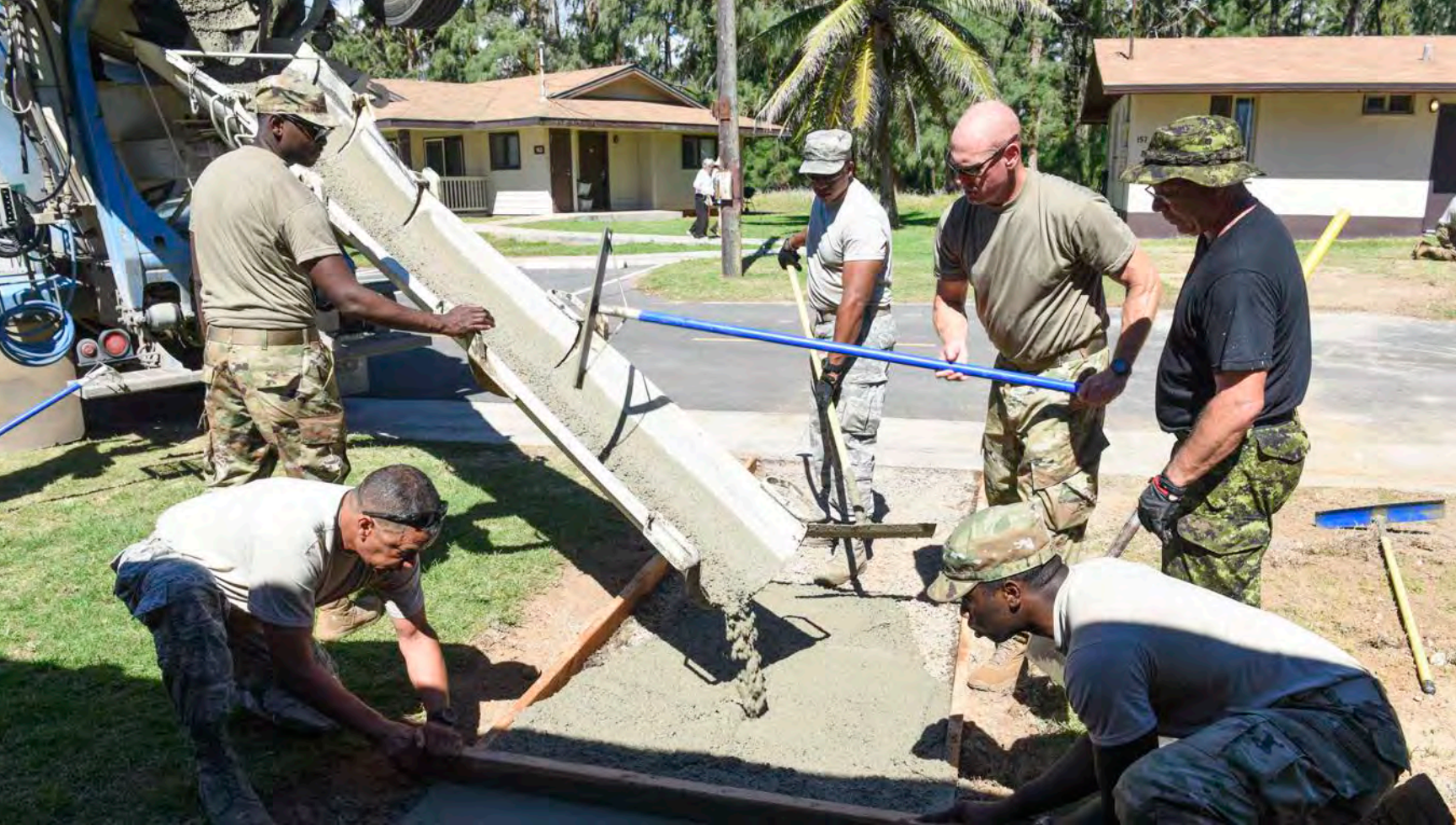
The South Carolina Air National Guard's 169th Civil Engineer Squadron, works alongside Royal Canadian Engineers from the 14 Wing of Greenwood, Nova Scotia, to pour and finish concrete sidewalks at the guest cabins at Bellows Air Force Station, Waimanalo, Hawaii.
